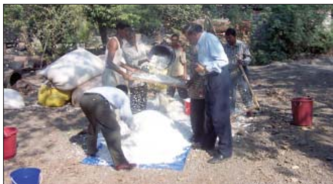
Screening of plastics waste to the required size
