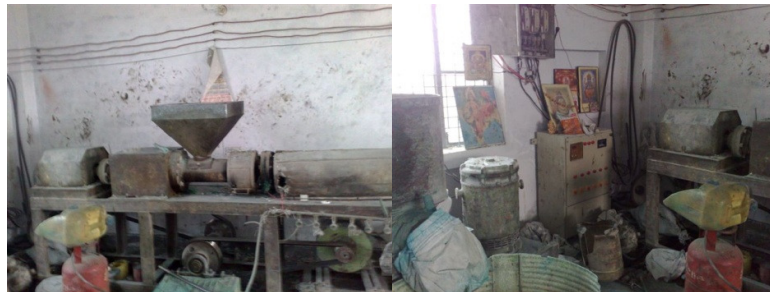
Inadequate Safety measures
