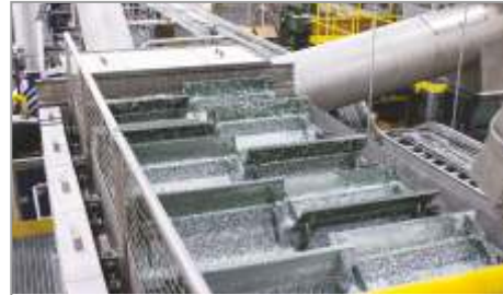
Figure 5 - Sink and Float Separator (Source - B+B Anlagenbau)
